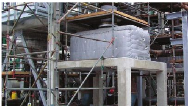
Figure 3: Alfa Laval Compabloc Welded Plate Heat Exchanger Installed in Vacuum Tower Bottom Steam Generation Service
