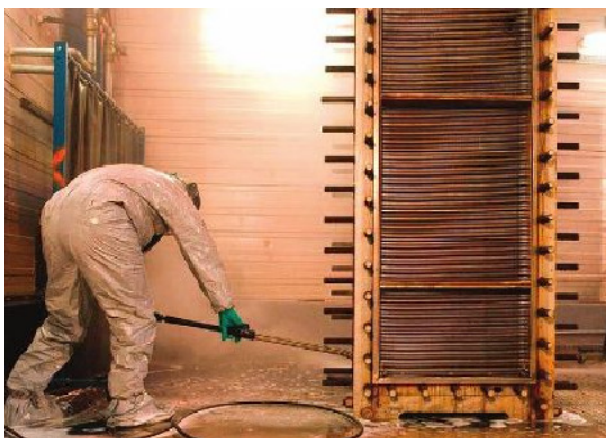
Figure 4: Welded Plate Heat Exchanger Cleaning with High-pressure Water
