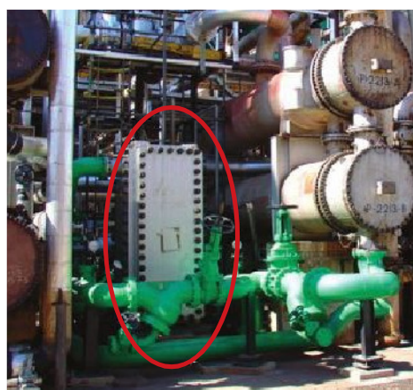
The single Compabloc welded plate heat exchanger circled replaced the two shell-and-tubes to the right.
