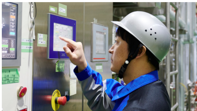
Mr. Jun Kubota adjusts parameters on the Alfa Laval De-alc control unit for a batch of low-alcohol beer at an Asahi Breweries production facility.
